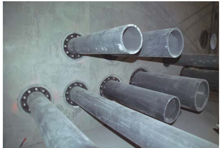
A combination of Century-Line® Sleeves and Link-Seal® Modular Seals perform a “No Leak Solution” for this pump room application.
